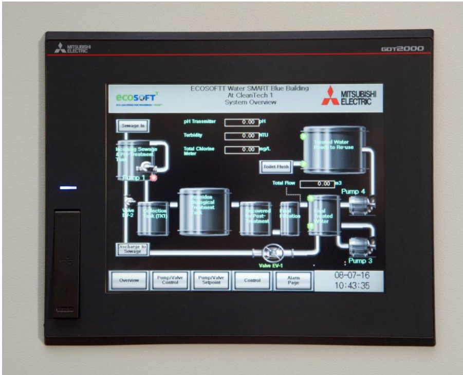
Caption: The easy-to-read interface provided by the onsite Human Machine Interface GOT2000 series gives administrators a clear window into the system's operation.
