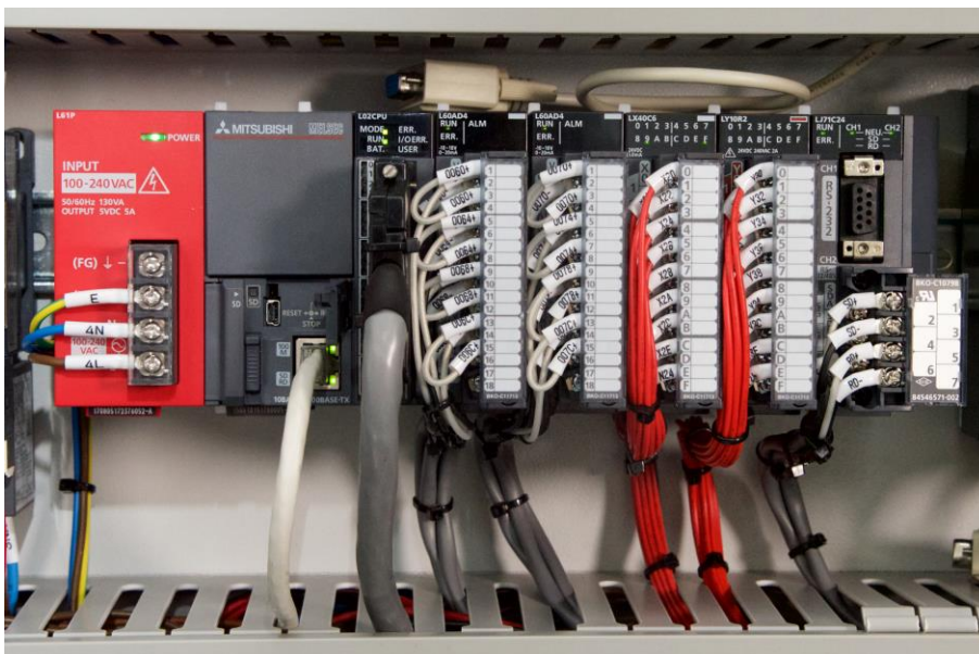
Caption: Mitsubishi Electric's L Series PLC controls complex processes for the wastewater treatment system.
